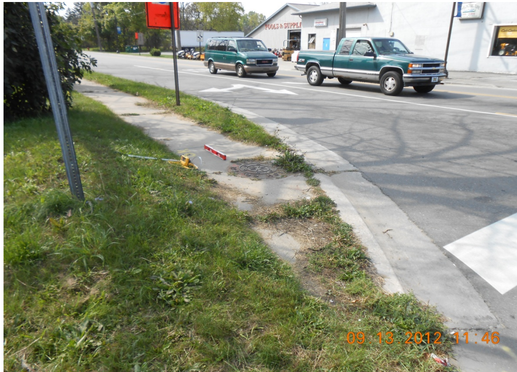
Picture 2: Crosswalk ramp on 32 nd Street at Lapeer Ave is in poor condition.
