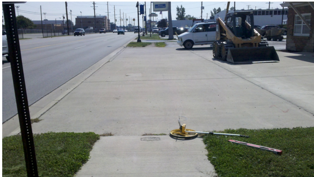
Picture 5: End of Existing sidewalk on 24 th Street, looking south on 24 th .
