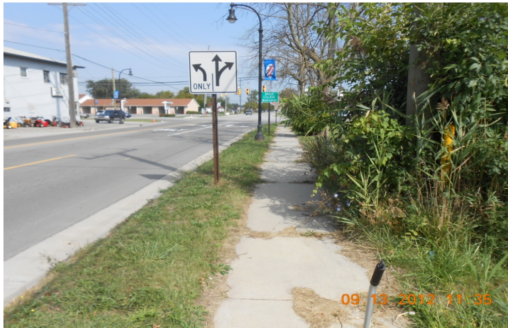
Picture 1: Sidewalk along 32 nd showing grass and weeds growing in joints and along side.
